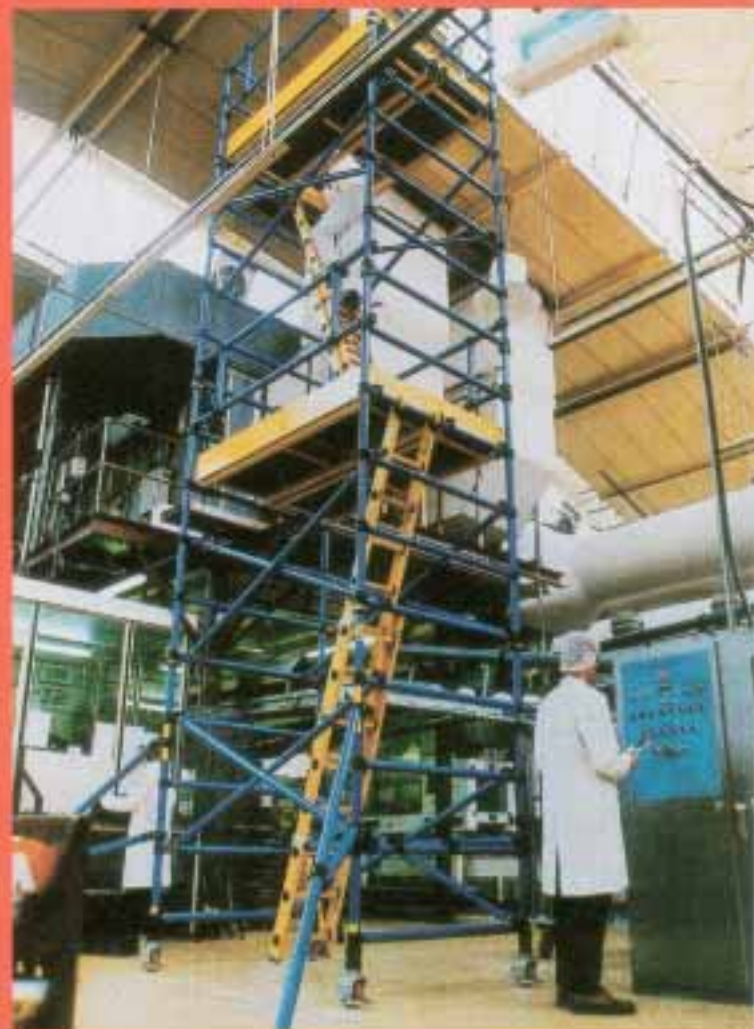
Inside maintenance with working system
